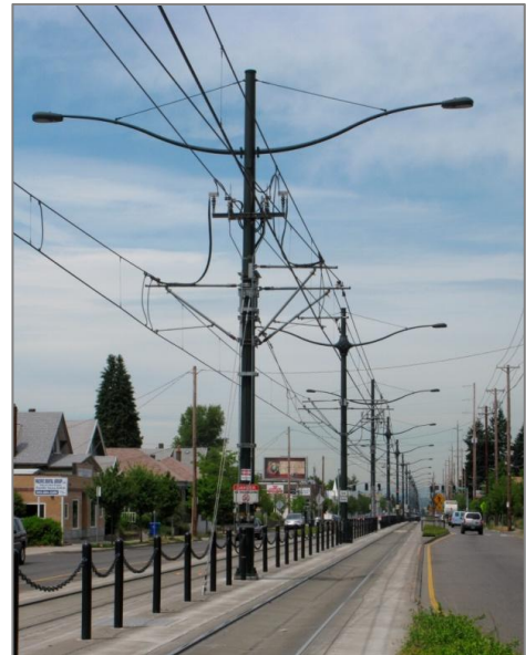
Joint use OCS/street lighting pole – Portland LRT
