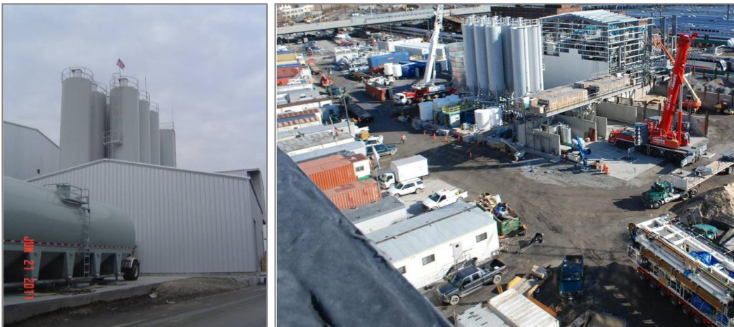
Typical TBM slurry plants and their associated operations
