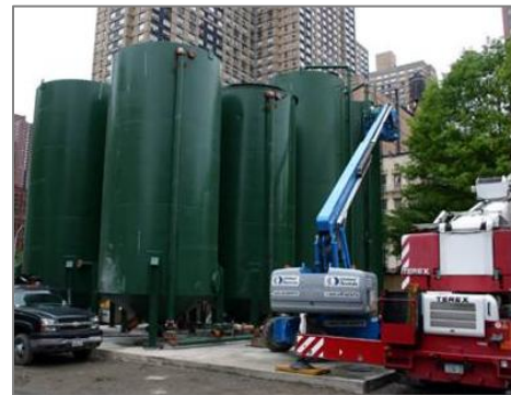
Typical Station Slurry Plant Equipment and Operations
